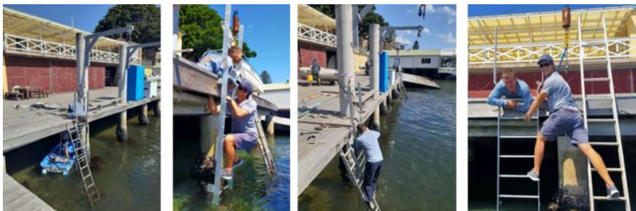
Club Captain Finn Irvine and handyman David Goldner installing the new stainless-steel ladders.
